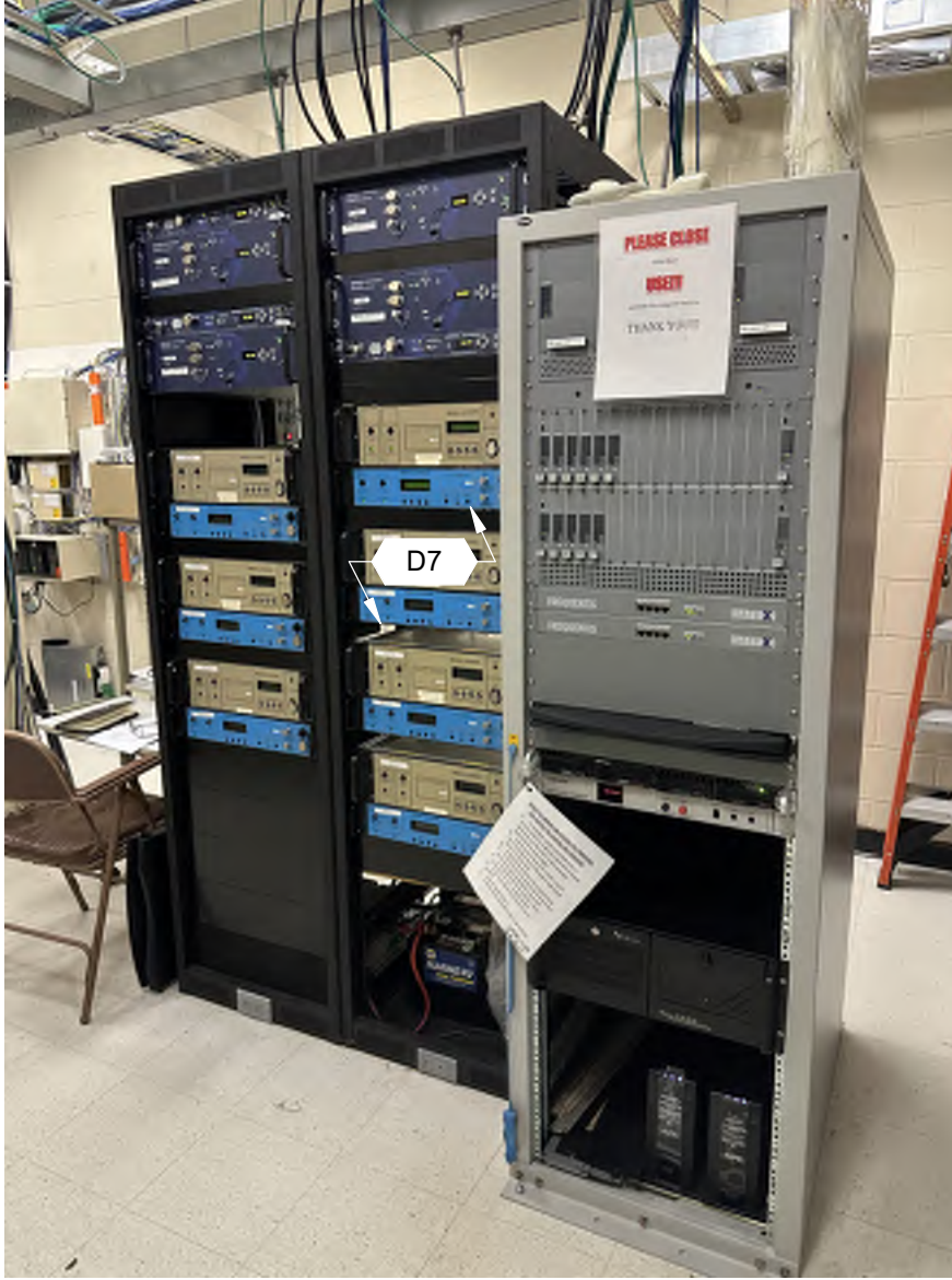
RADIO RACK IN THE EQUIPMENT ROOM
