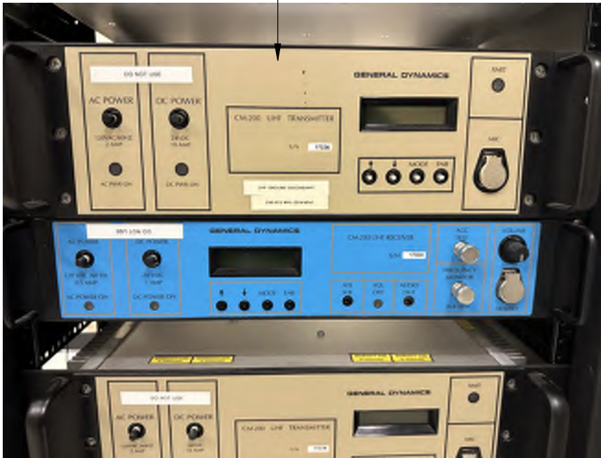
VHF GROUND SECONDARY RADIO (17236)
