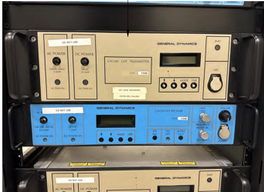
VHF GROUND SECONDARY RADIO (17235)
