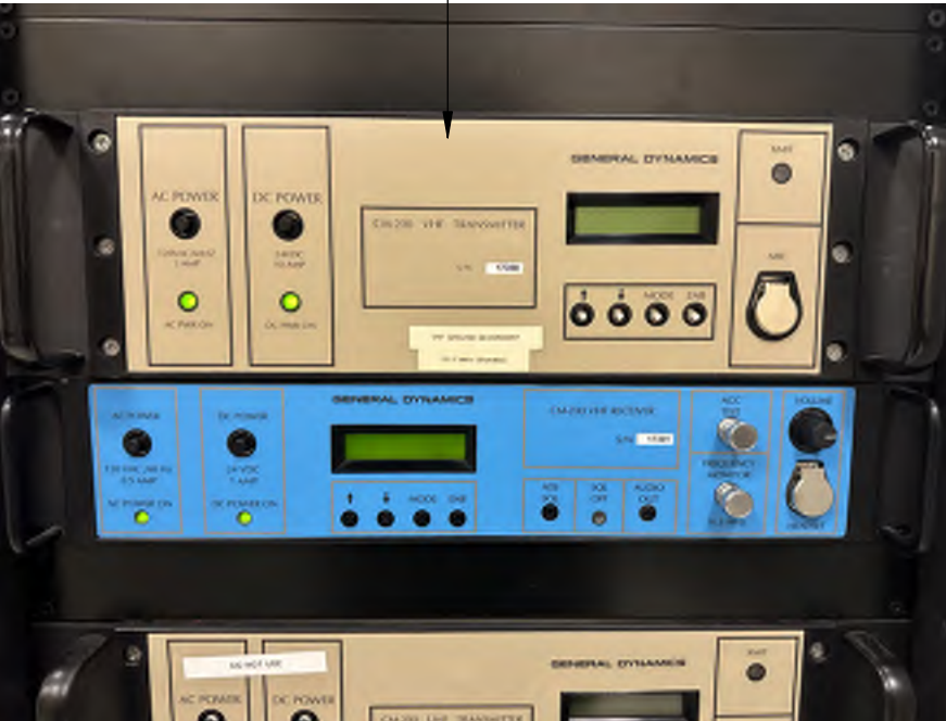
VHF GROUND SECONDARY RADIO (17390)
